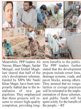
Meanwhile, PPP leaders Ali Nawaz, Bhao Magsi, Sardar Mengal, and Imdad Mughlani shared that half of the city's development schemes, funded by MPA Mir Nadir Khan Magsi, have been temporarily halted due to the installation of new gas pipelines. They emphasized that these projects will resume to ensure high-quality completion, providing long-term benefits to the public. The PPP leaders further stated that the development projects include sewer lines, drainage systems, roads, and paver blocks, among others. They assured that no irregularities or corrupt practices will be tolerated in the implementation of these schemes, and public funds will be spent solely for the benefit of the people.—RT
