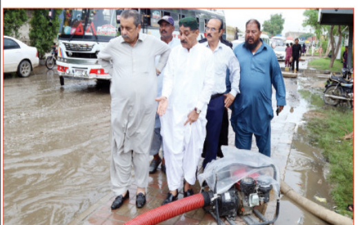
KARACHI: Advisor to the Sindh CM Syed Najmi Alam and Chairman of Malir Town Jan Muhammad Baloch are inspecting the rainwater drainage work on the National Highway near Popular Factory. —Photo by Asif Qureshi
