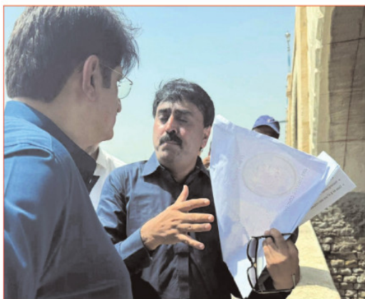
SUKKUR: Sindh Chief Minister Syed Murad Ali Shah is inspecting the repair work of the Sukkur Barrage's Gate No. 47 and 44 which had been severely damaged.-RT
